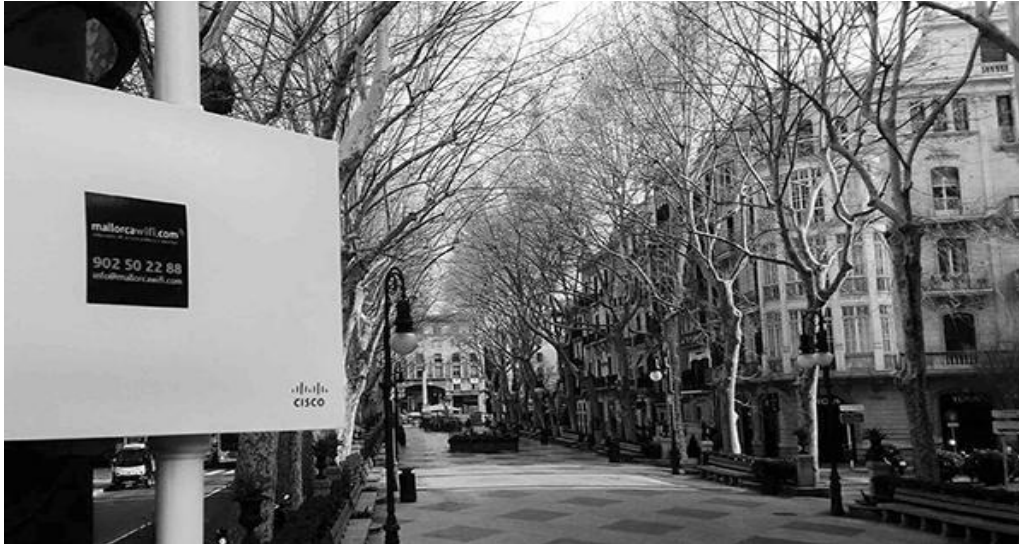
Figure 1. Wi-Fi Access Point installed in Paseo del Borne from Palma City
